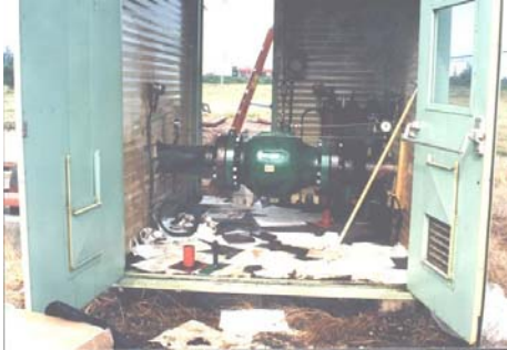
Relief valve and instrumentation enclosure.
